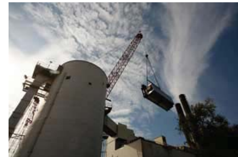
Indiana University’s Central Heating Plant (top) was renovated in 2009 to function more efficiently. New boilers and filters along with lime and carbon-flue gas injection systems reduce emissions and particulate matter that pollute the atmosphere. Photo Credits: IU Photography
